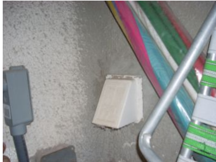
Dryer vents to enclosed closet
