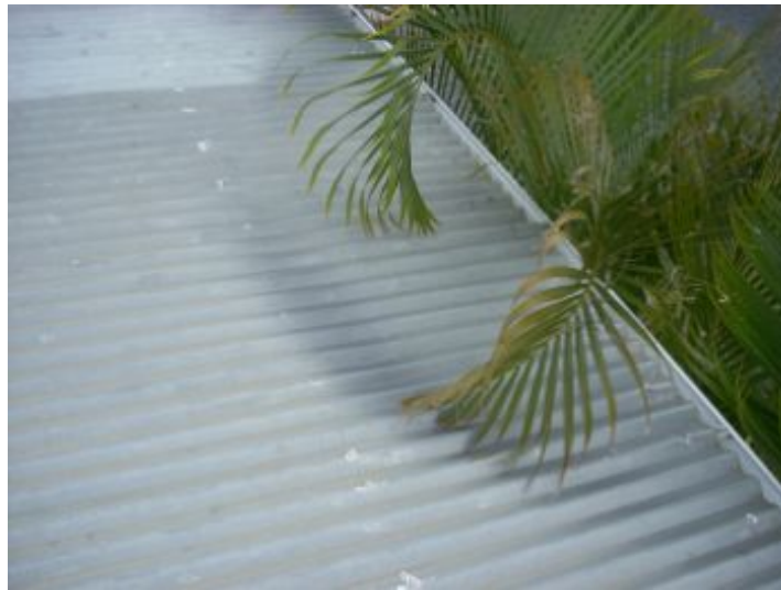
Trees overhanging roof should be trimed back
