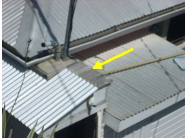
Bare plywood on this surface
