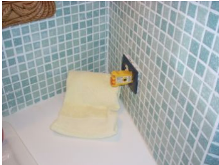
No GFCI in Master Bath
