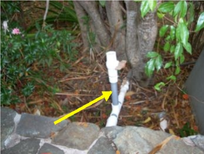
Supply line for hot tub made with electrical (gray) PVC
