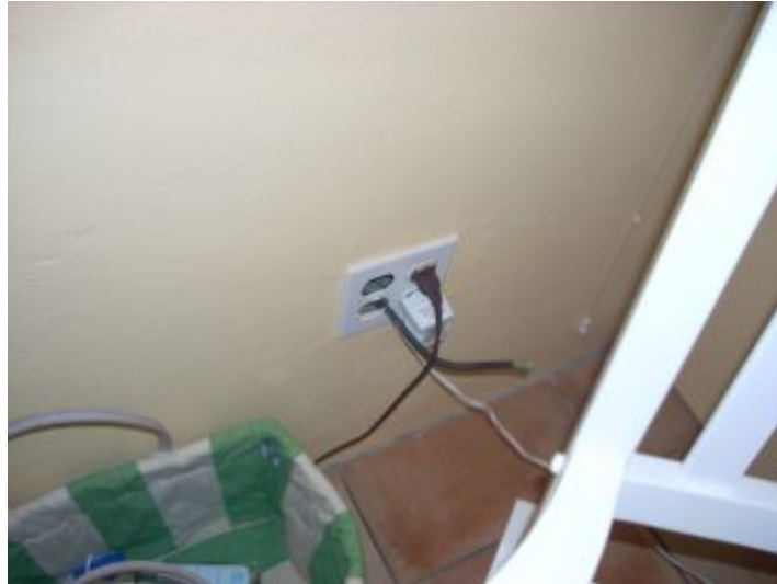
Cable (low voltage) and 110v in same junction box
