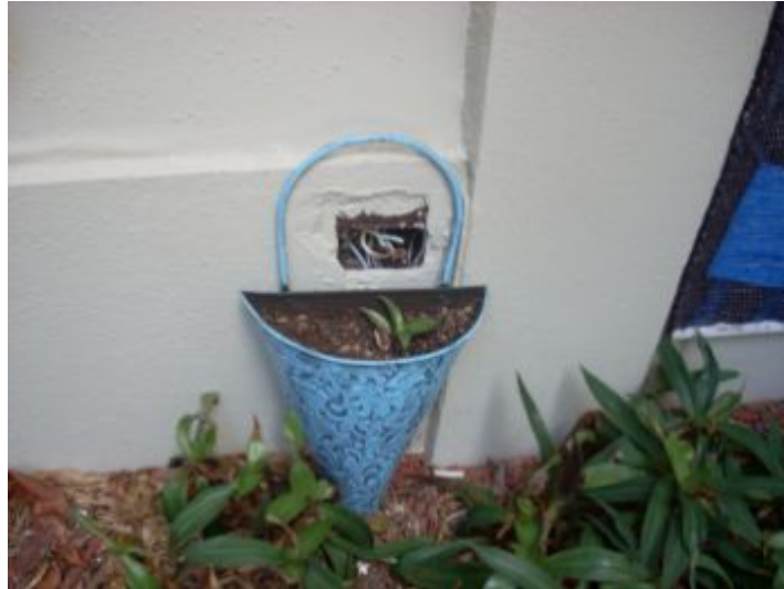
Missing cover on junction box
