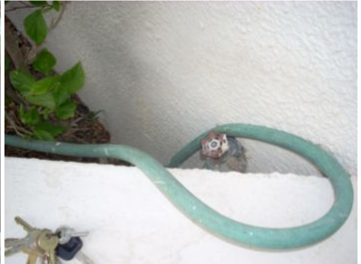
Hose bib at front of house
