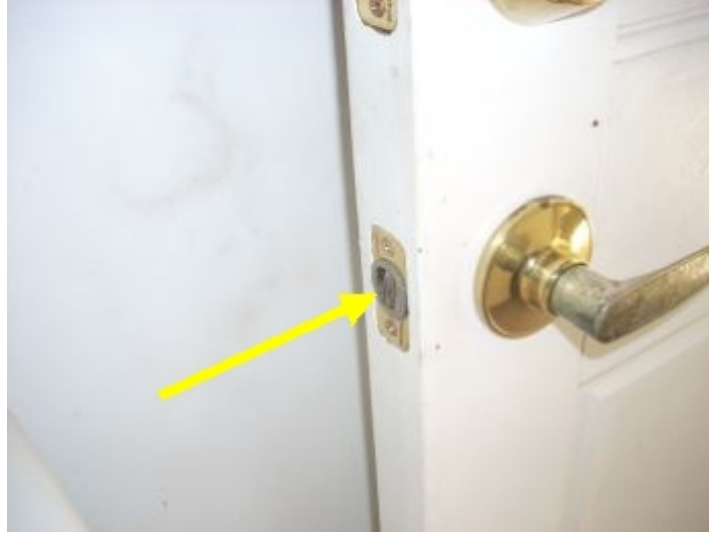
Kitchen door striker is stuck
