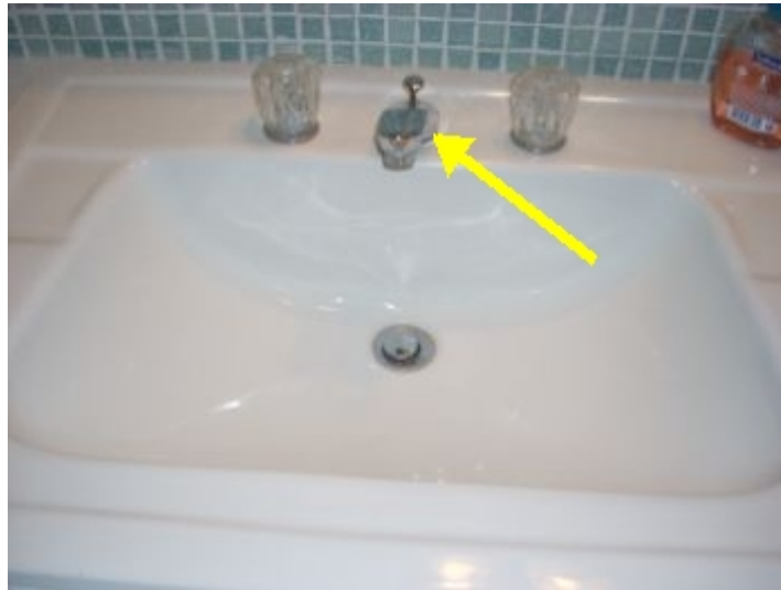
Faucet is loose
